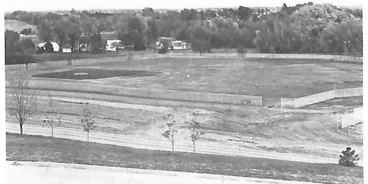
Construction is underway on the baseball field, part of the new sports area.
