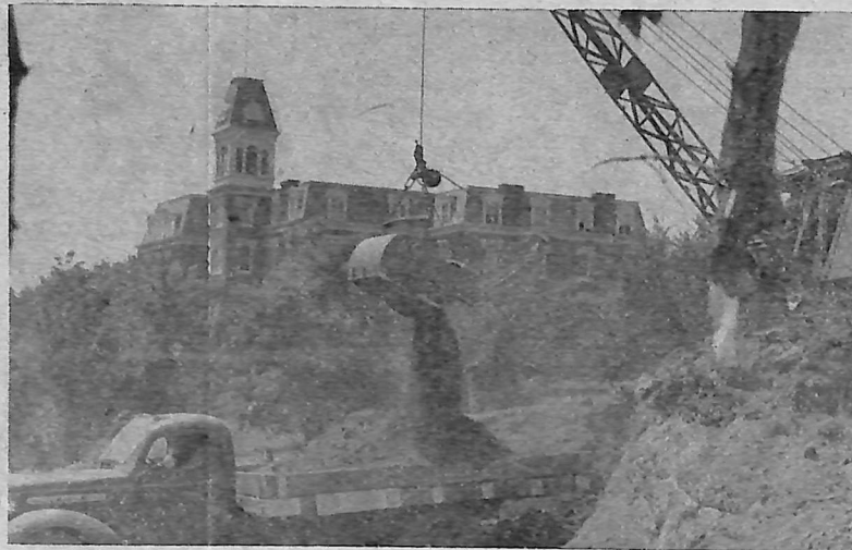
This was the scene on Dana Hill in the month of August as the first load of dirt was being hauled away from the excavation for the new building.
