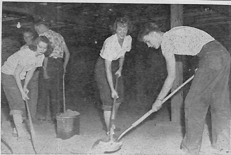
Three ambitious students are shown here helping level the ground in the gymnasium basement in preparation for laying the concrete which was recently completed.
