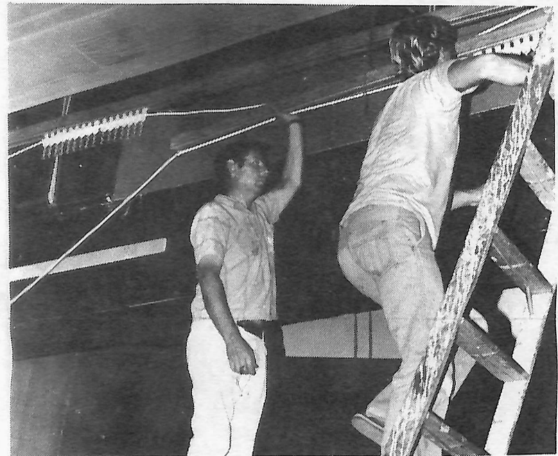
Hanging stage curtains is quite different from hanging curtains in a home. Mr. Sieghard Krueger directs Alpha Psi member Tim Nietfeld, '80 in hanging the curtain. Also involved in the renovation were such projects as painting and replastering.
