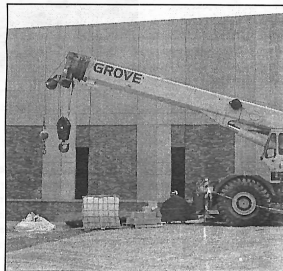
Construction on the Borup Coliseum addition will conclude in the summer of 2003. Photo by Lysnie Cetto.
