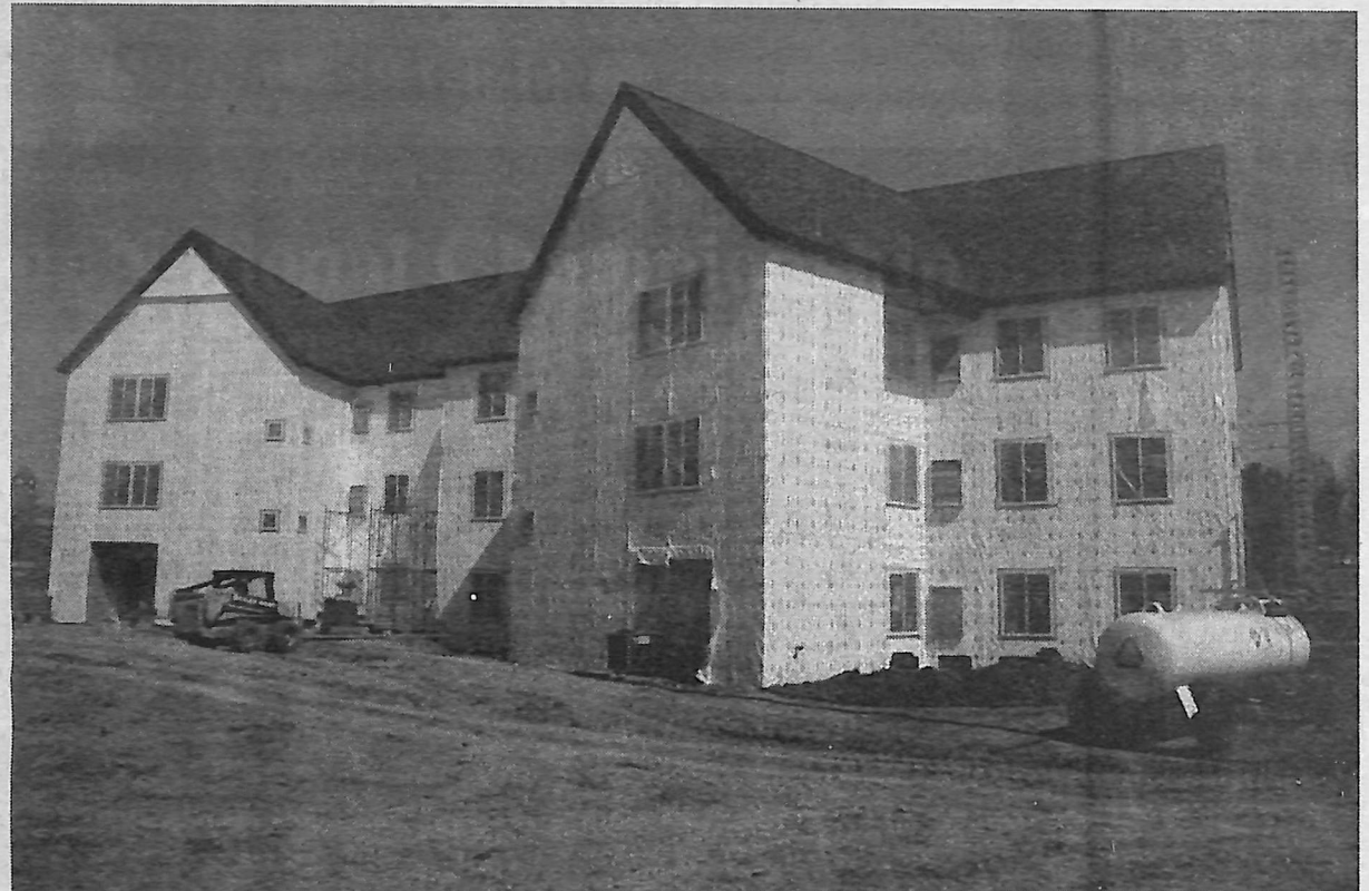
Exterior brick laying and interior cabinetry work has begun on the newest residence hall on the Dana College campus. The hall will be open for student housing this fall.
