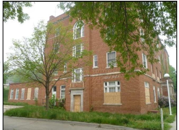
Argo Hall shows the typical campus-wide deterioration that has taken place since the campus was vacated six years ago.
